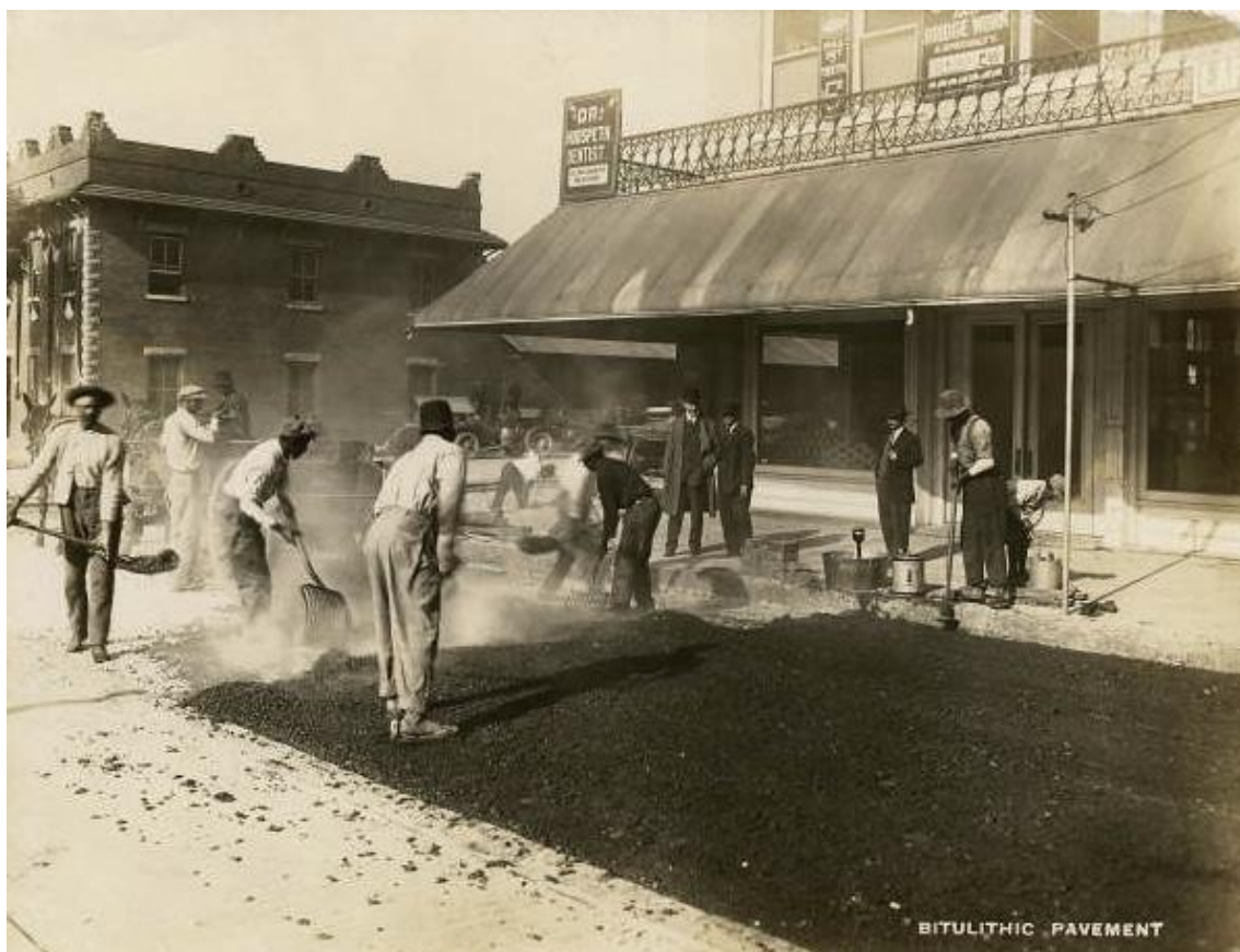
Road construction workers laying bitulithic pavement. 1920 ca. Florida Memory . Document en el domini públic.
